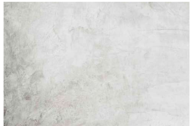
DIRTY/OFF-WHITE STUCCO FINISH
