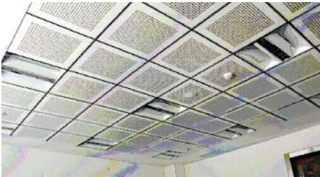
RCP-C 600X600 ACOUSTIC BOARD CEILING WITH SQUARE TROFFER LIGHTING
